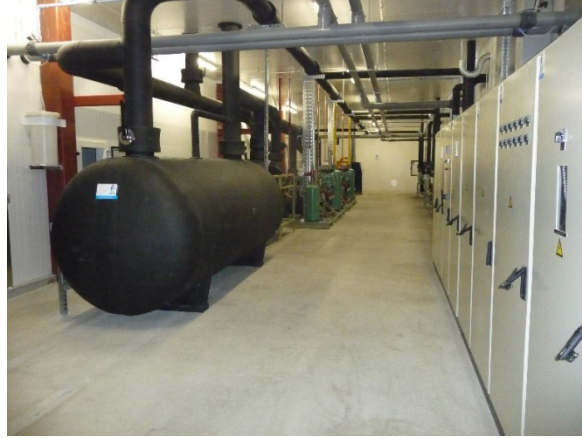
Accumulation vessel for the glycol
