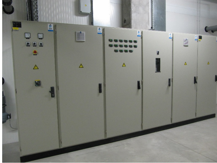
Main electrical switchboards
