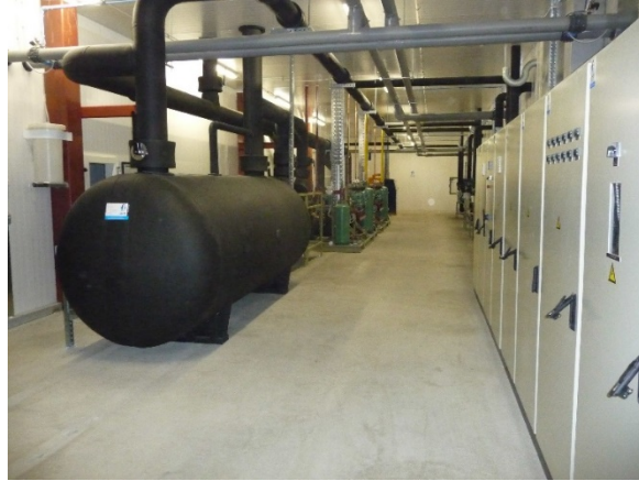
Accumulation vessel for the glycol
