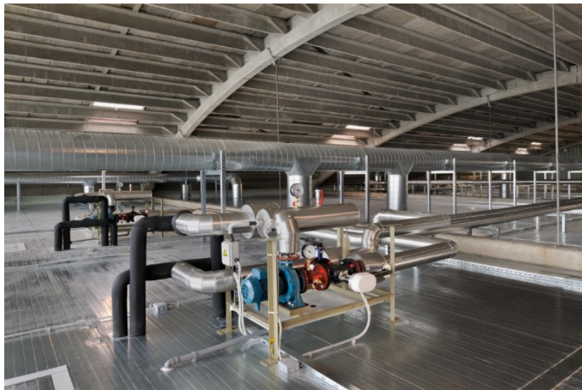
Pump stations with control valves and pumps
