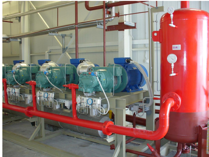
Refrigeration unit with screw compressors
