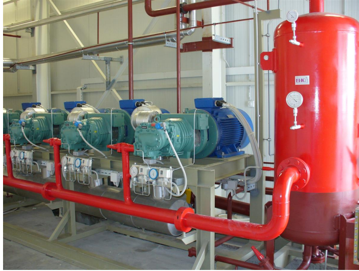
Refrigeration unit with screw compressors
